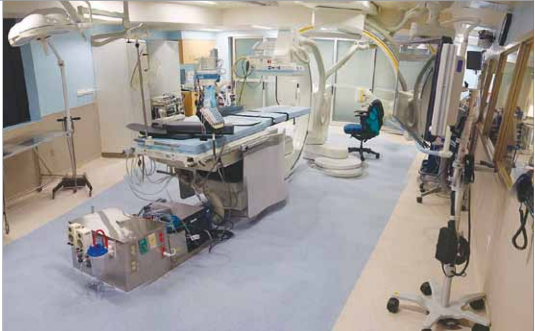
Right: This newly renovated Electrophysiology Lab is used for treating heart rhythm disorders.
